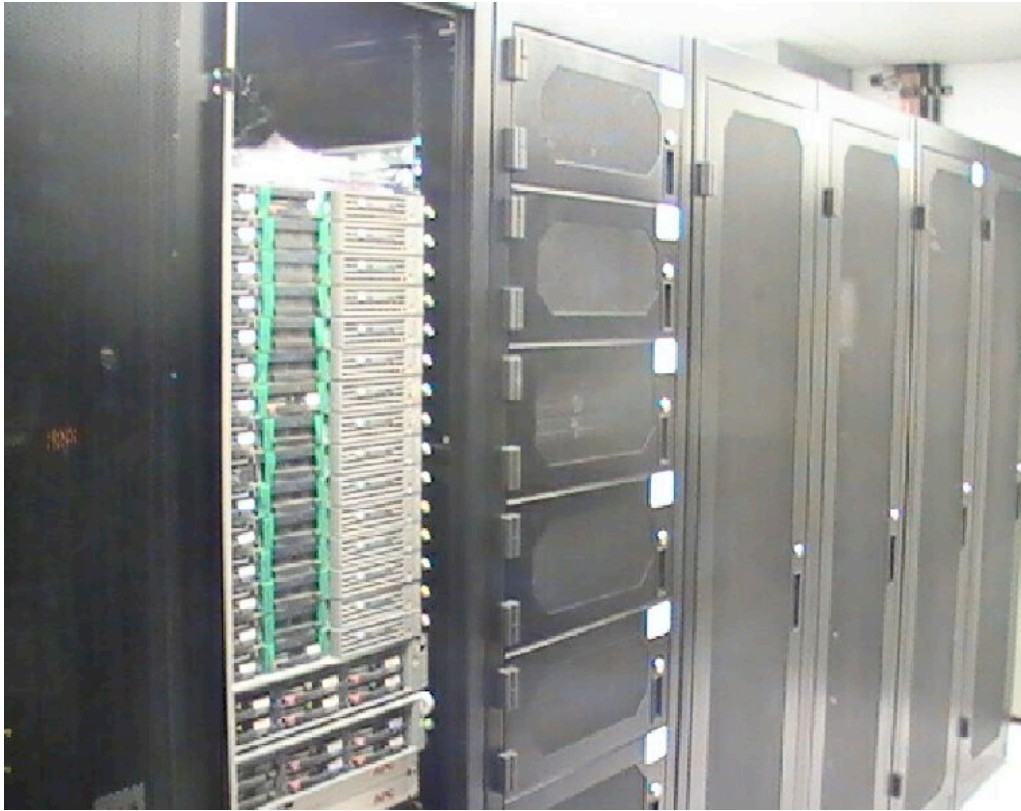
Figure 1. Rack Server – (In white above) Fifteen 1U blade servers on top of two 2U blade servers and two 1U UPS
